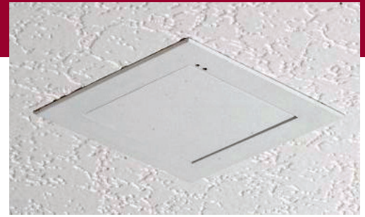
Installed View (Normal Mode)
